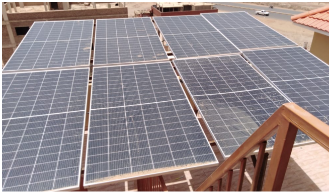
Fig. 4. Solar Panels Orientation for optimum power generation (Khartoum, Sudan)
