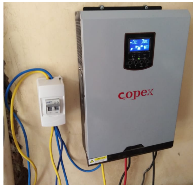
Fig. 3. Copex Solar Power Inverter
